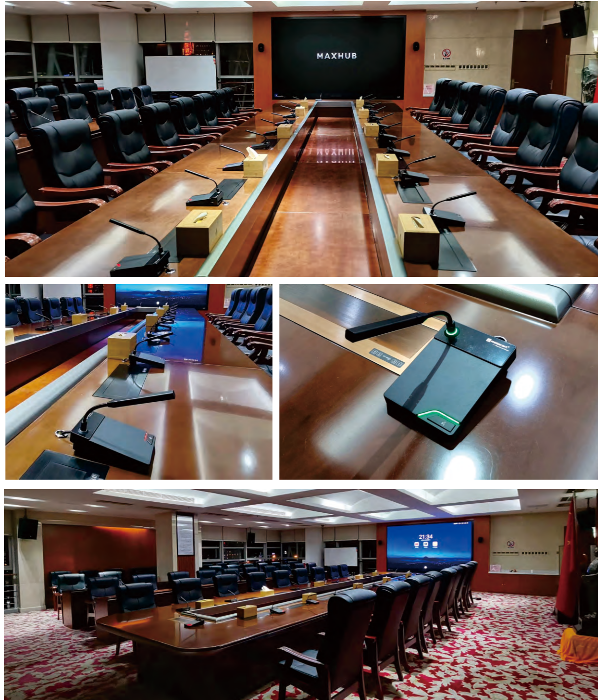
CS-302+CS-501+EU-610 | CS-302 wired professional digital conference and discussion system is stationed in the conference room of the Standing Committee of Tianyuan District
