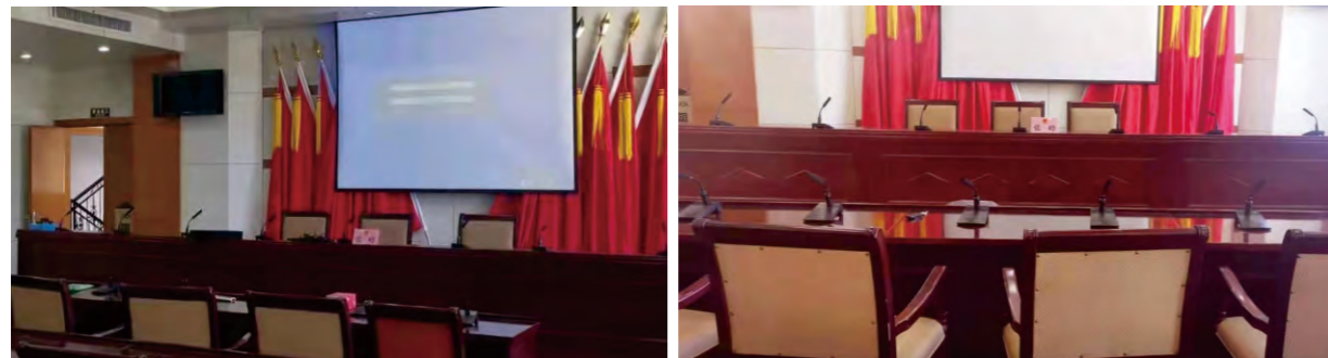
WDC-903 | WDC-903 digital wireless conference and discussion system is installed in a multi--functional conference hall of a municipal government department
