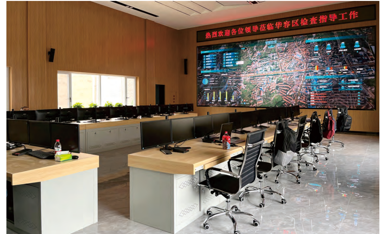
UR-222DMB+UR-111DMH +CS-302+CS-501 | Replace and upgrade the conference system of digital rural command Center in Huarong District
